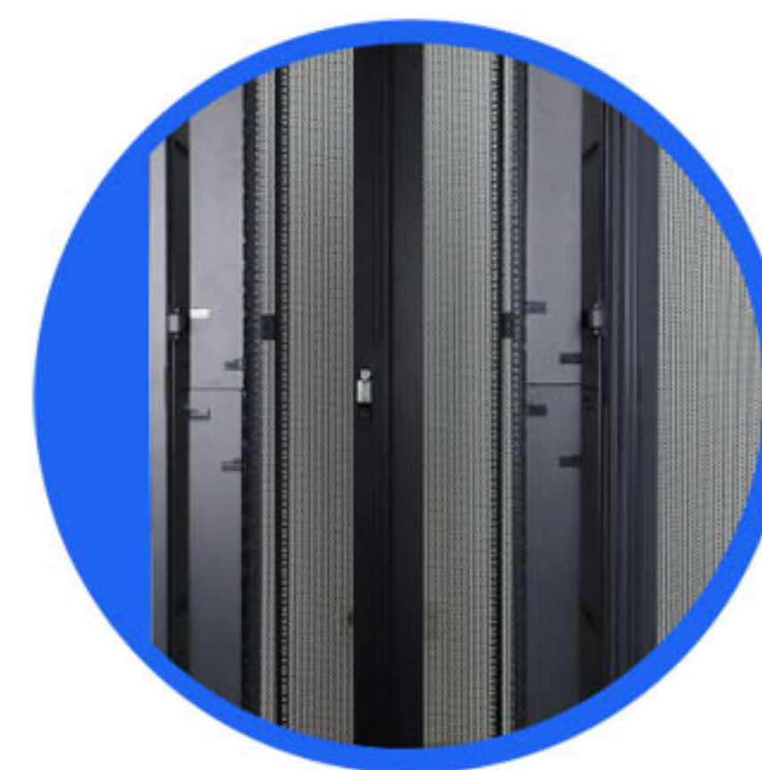
Vertical Cable Duct
